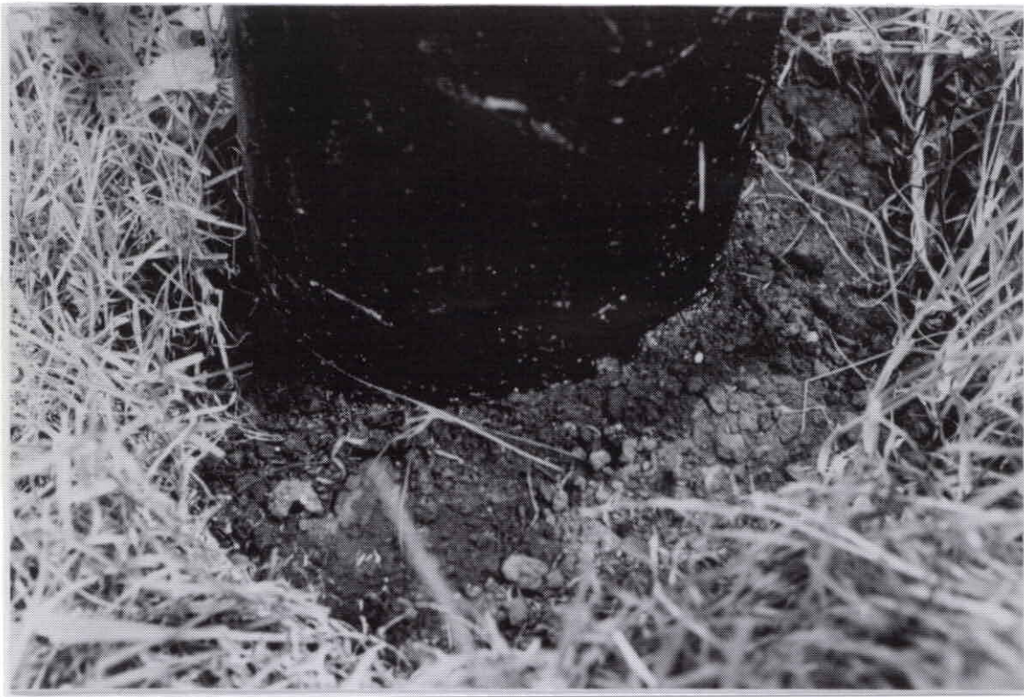
Fig. 1. Ground line of standard transmission pole (treated with 100\text{kg.m}^{-3} creosote by the full cell process) after 12 months' service . Bleeding creosote is visible running down the surface of the pole and the soil surrounding the pole is visibly polluted with the leached creosote. Note lack of vegetation in bare polluted zone of poisoned soil.
